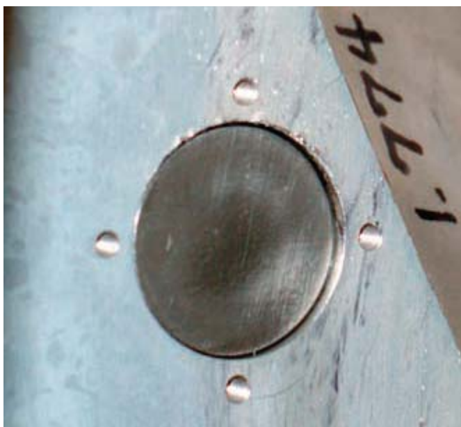
Figure 4 The sensor pocket fitted in the fan casing
